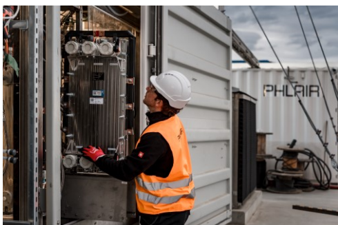
Blick in den Technikraum von Phlairs DAC-Pilotanlage in Kanada. Copyright: Phlair.
